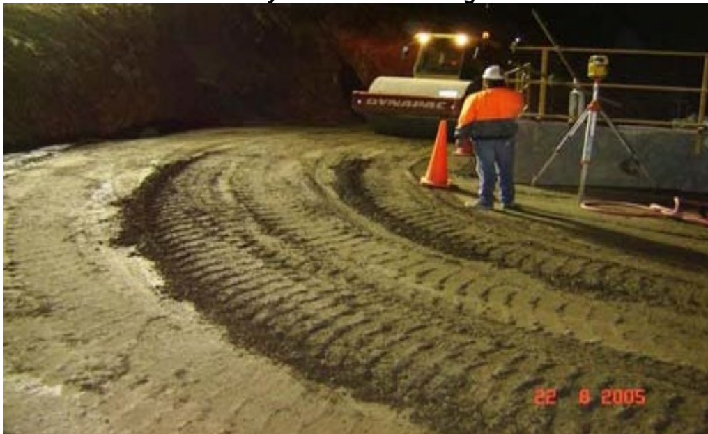
PICTURE 2. Surface damage (RL 73.315) on access during placement Of 2nd layer to RL 73.625 - Nightshift
